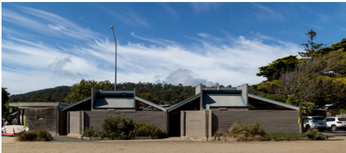
The aging toilet block at Grove Road in Lorne is ready for a complete refurbishment in 2024.
